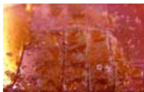
Peel-off was observed across the sample substrate.
