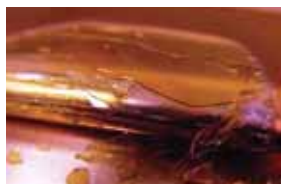
Major peel-off was observed.
